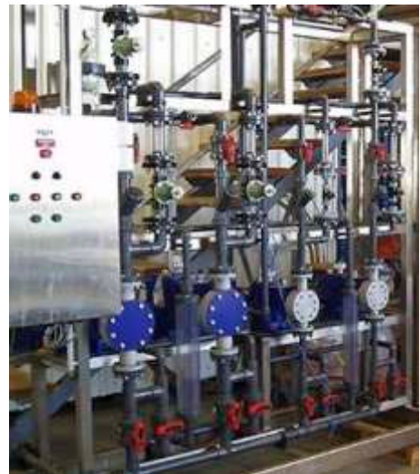
Chemical dosing system
